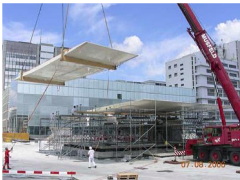
Figure 1: Multifunctional sandwich structure for the roof of Novartis Campus Main Entrance Building (Basel, CH).
